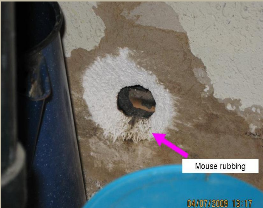
Mouse rubbing on entrance to opening in drywall Image Credit: Daniel F. Hoyt, GRIC EHS
